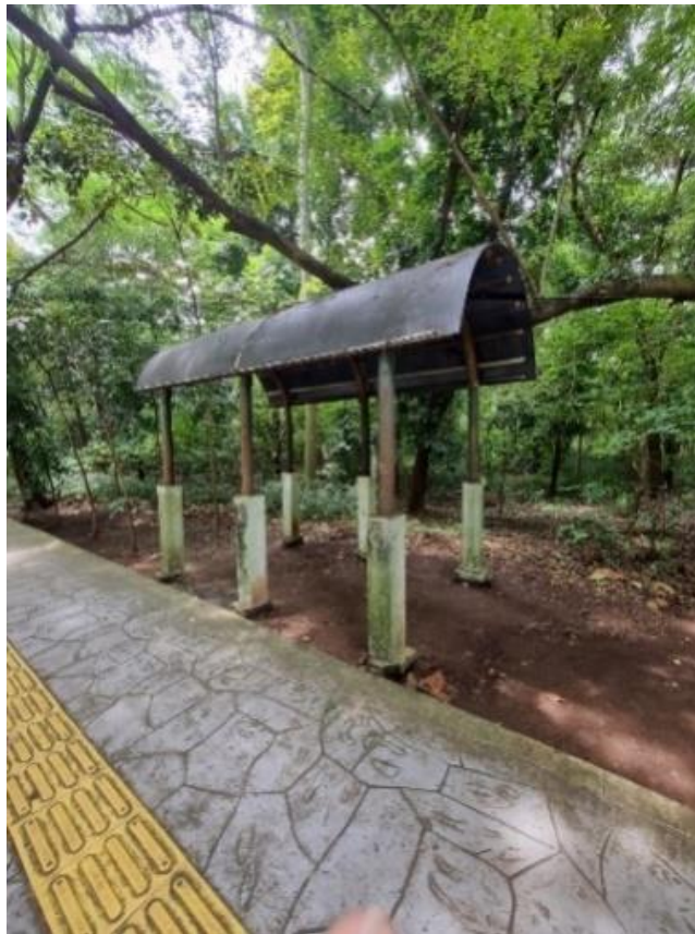
Picture 6. Shelters that need to be renovated
