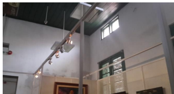
Figure 3 Windows and Vent Opening with White Steel Partition In Museum of Fine Art and Ceramic (Source: Wulandari et al. , 2016)
